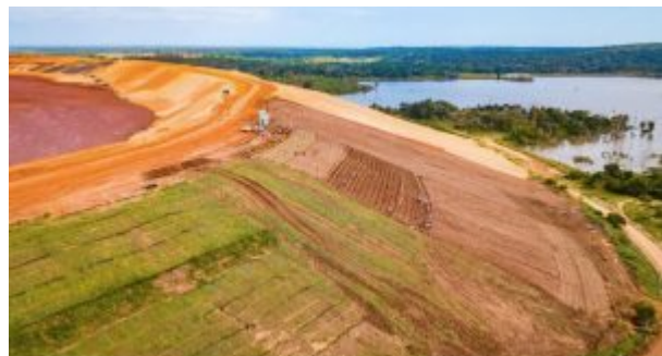
Rehabilitation works at the TSF with the Mukurumudi Dam in the background
